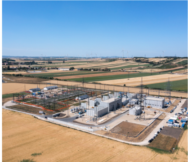
A new substation in Neusiedl an der Zaya was also built as part of the project.
