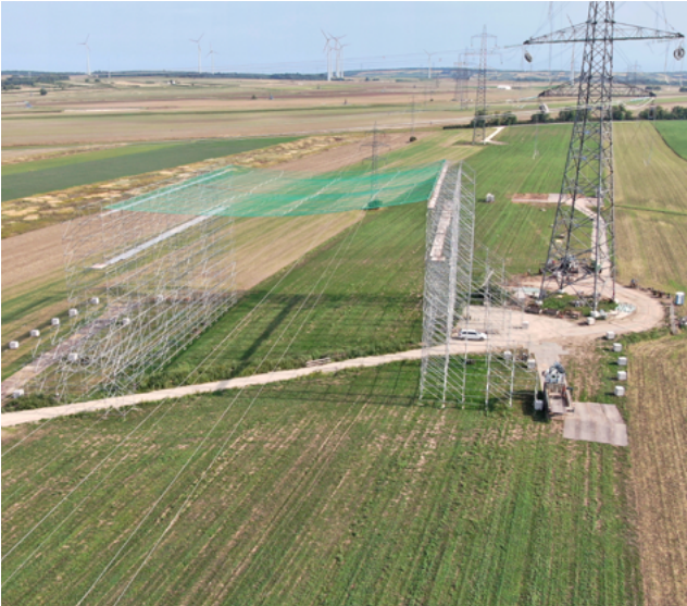
The new Weinviertel line includes 202 pylons, each of which is around 60 metres high.
