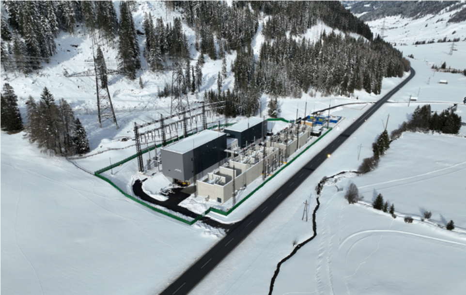
Commissioning of the Nauders substation: The Reschen Pass project was completed on schedule in December 2023.
